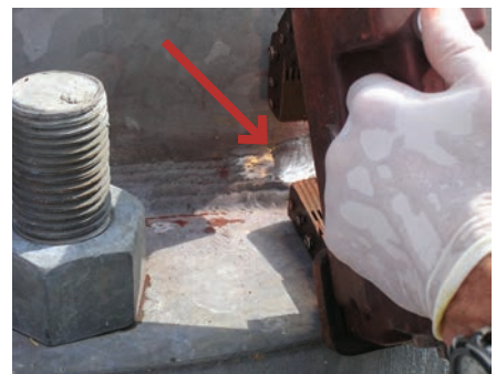
Figure 10. An MT exam showing indication (crack) at upper toe.
