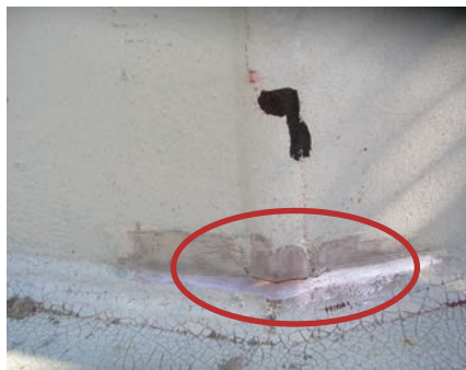
Figure 9. A toe crack is still visible via MT exam after grinding.
