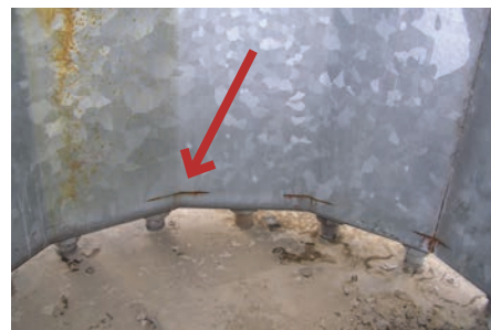
Figure 11. Socket-style pole base through-wall toe cracking viewed from the inside of the pole (visible rust).
