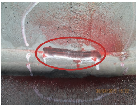
Figure 8. A minor toe crack is visible via MT powder after light grinding.
