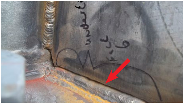
Monopole Base Plate Stiffener Underfill
