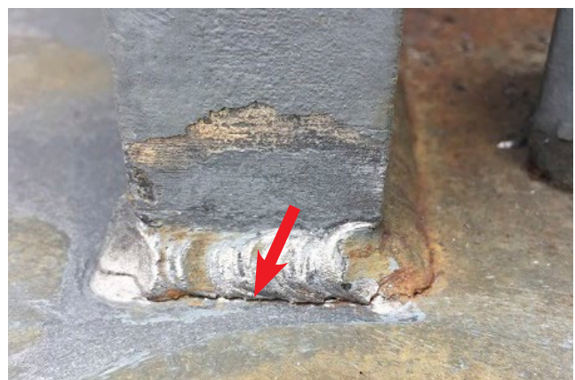
Base Plate Stiffener Weld Lower Toe Crack
