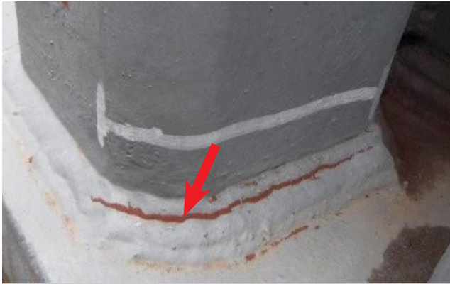
Anchor Rod Bracket Longitudinal Crack (Shown in Red)
