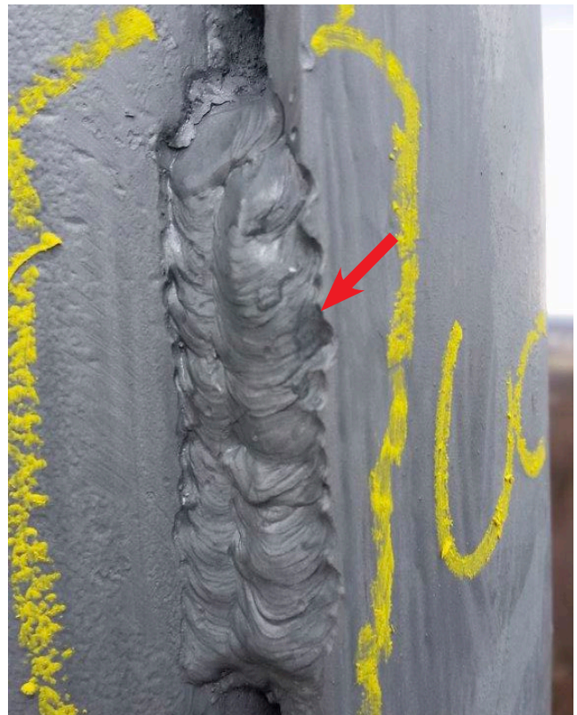
Tower Leg Split Pipe Stitch Weld Undercut
