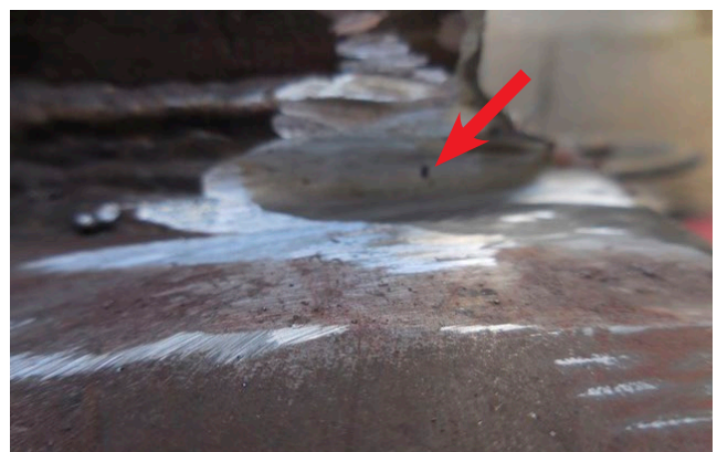
Monopole Base Plate Stiffener Weld CJP Connection Slag Inclusion
