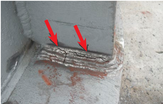
Stiffener Longitudinal & Transverse Cracks (in Black)
