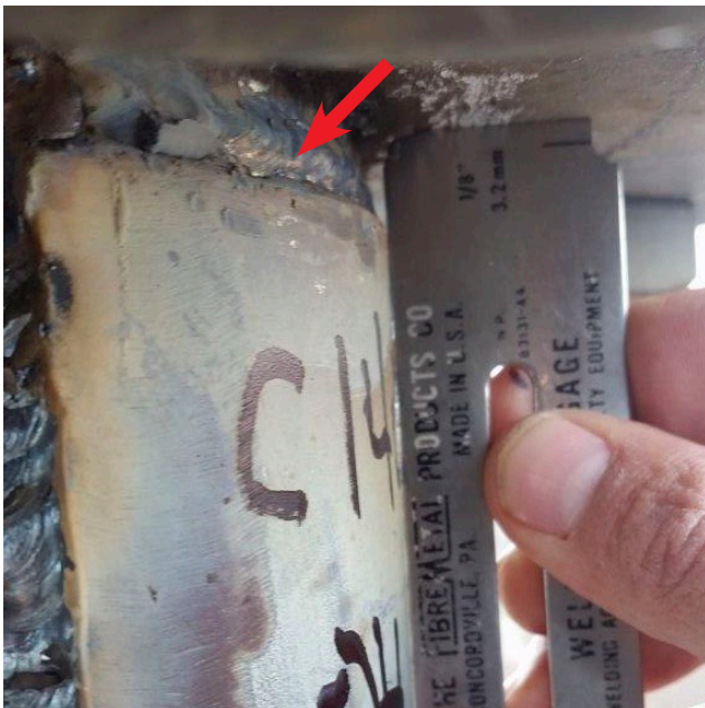
Tower Leg Split Pipe Modification Incomplete Joint Penetration to Leg Flange
