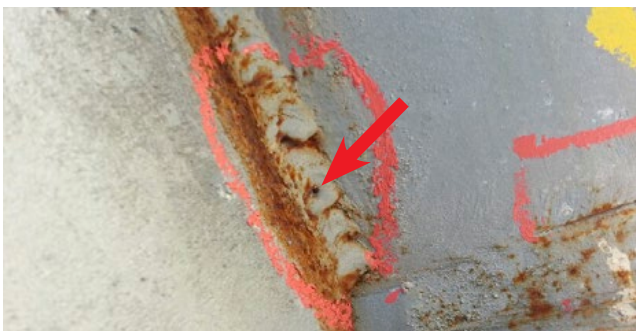
Examples of Porosity in Monopole Modification Welding
