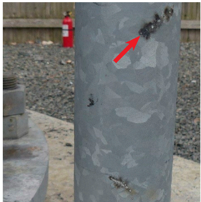
Arc Strikes on Ice Bridge Post
