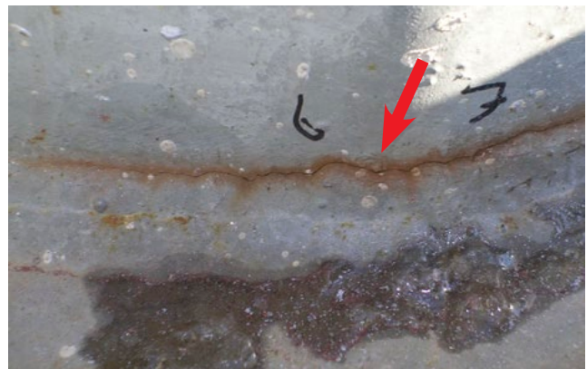
Monopole Base Plate Weld Upper Toe Crack
