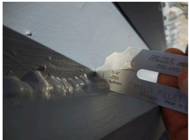
Required Stiffener/Plate Modification 1/4" Fillet Welds Undersized by Fillet Weld Gauge Measurement
